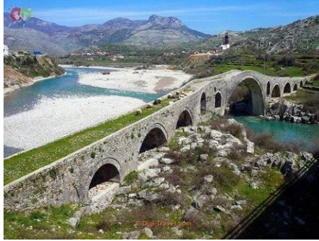
Figure 25. Mes Bridge (Ura e Mesita) on the Kir river, near Shkoder, Albania (1770)
